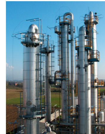
Fig. 8. The appearance of the distillation column
